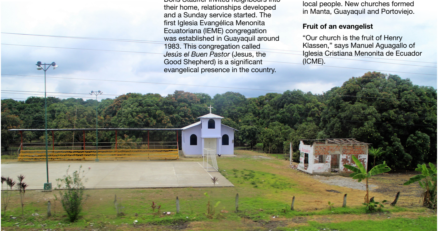
A church in an earthquake damaged region of Ecuador after 2016.
