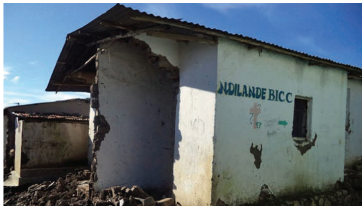
The Ndirande Brethren in Christ church building, damaged by heavy rainfall in January 2015. According to a report by Rev. Francis Kamoto, the building’s sanctuary was saved from destruction, though other parts of the structure were destroyed.
